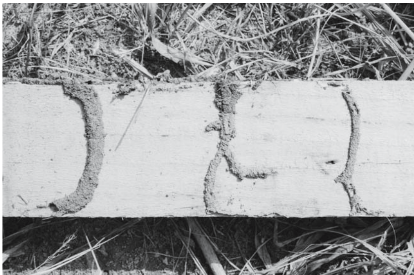
Figure 7.4 Termite earthen tunnel across a treated wawa board. The narrow tunnel often indicates this is a transport tunnel
