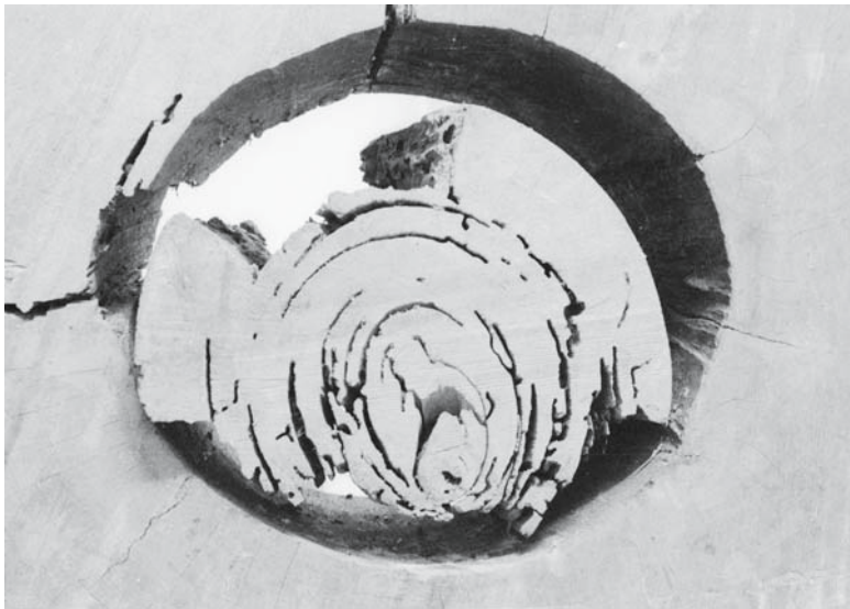
Figure 7.10 Coptotermes caused damage to the center heartwood of a living Khaya sp.
