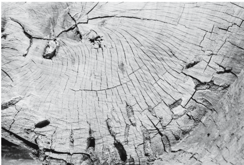
Figure 6.8 Mature longhorned wood borer larvae will often excavate tunnels into the wood
