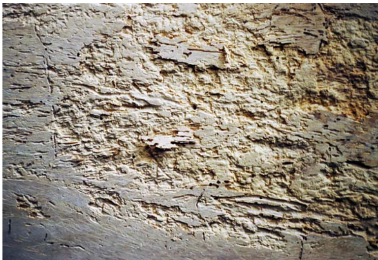
Plate 56 Surface view of powder post beetle damage to wawa.
