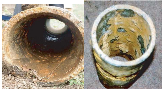
Figure 4.32. Old cast iron pipes.
