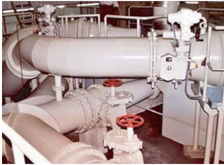
Figure 4.76. Piping in pumping station.
