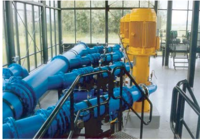
Figure 4.78. Unmanned booster pumping station.
