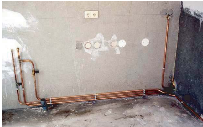
Figure 4.38. Indoor installations made of copper.
