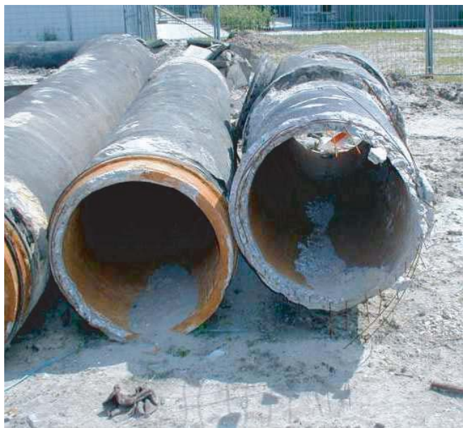
Figure 4.39. Old concrete pipes reinforced with steel net.
